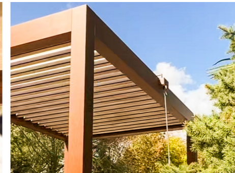
The installation of the accessories that will open and close the panel profiles is completed.
