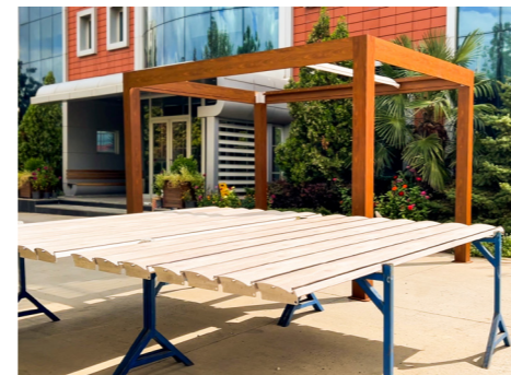
The panel profiles that will provide shading are removed from their packaging.
